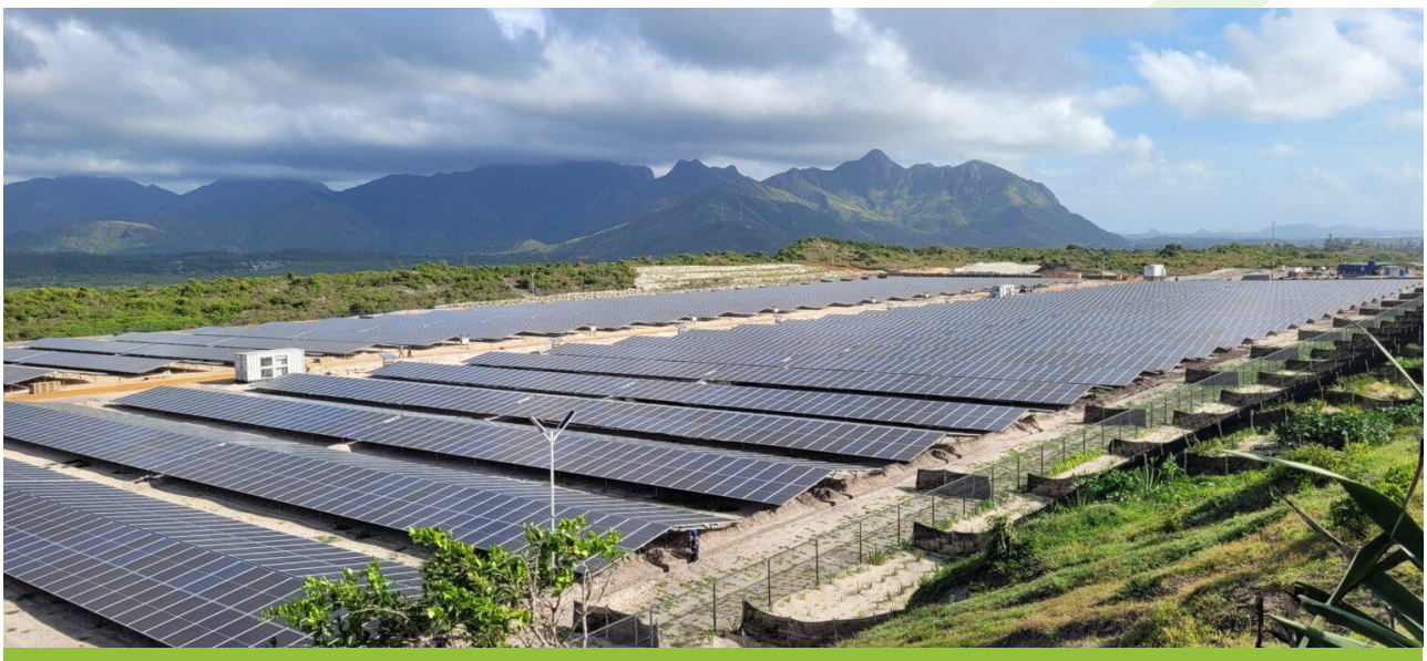
Figure 19: CrossBoundary Energy's QMM hybridised project. Source: GWEC market intelligence 2023
