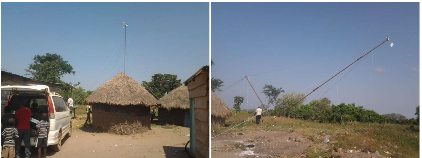
Photos above were taken during installation of the wind turbine at Lufudu site in 2014
