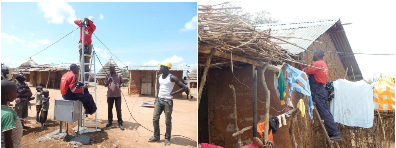
Photos above show installation of cables and wires to peoples' houses in Lokopo in 2015
